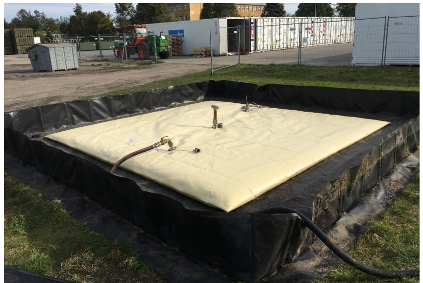
Overseas Military Supply Base 11-site 33,000 gal. fuel installation
