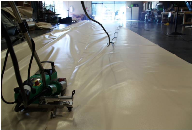
DLA — Dry Dock Containment Liners SPMYM2-17-P-1096, SPMYM2-16-M-2361
