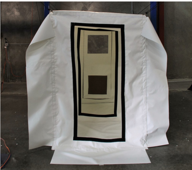
Puget Sound Naval Shipyard Worker Safety Containment Room
